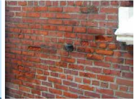
Deterioration of brick caused by moisture is marked by discoloration and brick erosion.
