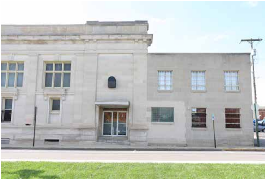
This photo shows the elements of continuity in brick bands and matching elevation of this urban infill's side façade. The addition houses additional office space, with the newer windows aligning with the historic windows but not completely matching in size or style
