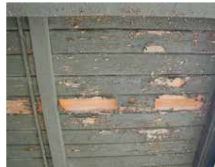
Paint failure on the underside of a wood canopy.
