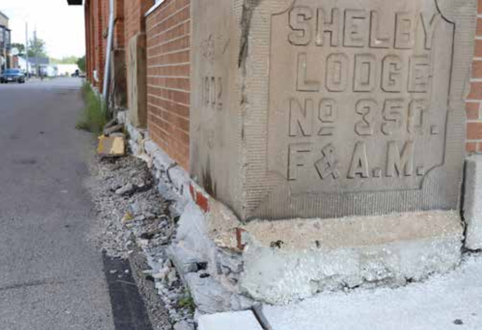
Foundations may exhibit efflorescence as a result of damage from salt-based snow removal chemicals.
