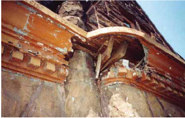
A painted lead-coated copper cornice is missing elements due to advanced deterioration of metal.
