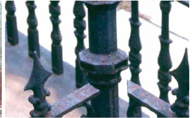
A corroded metal fence has failed at the connections between the railings and the post.
