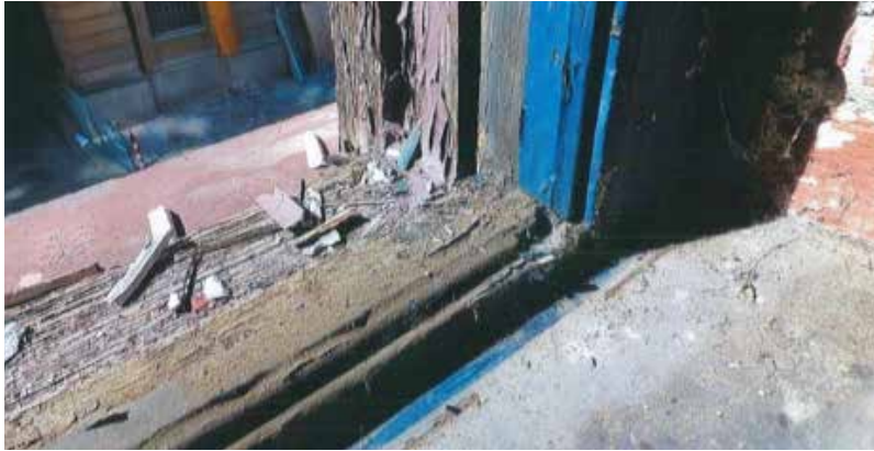
This photograph shows a window sill damaged beyond repair.
