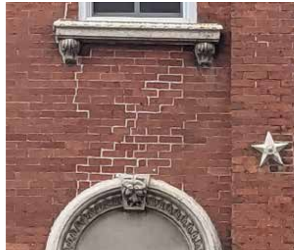
Incorrect use of mortar can impact the aesthetics and character of a building.
