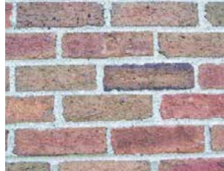
Damage to brick caused by sandblasting.
