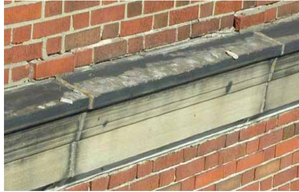
A loose stone cornice attached by metal fasteners indicates that its fasteners have failed.
