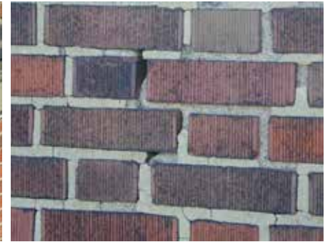
Previous poor repointing. Repointing mortar is deteriorating due to improper execution.
