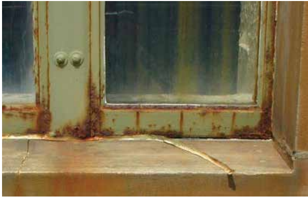
Corrosion/rust on a steel window sash resulting from exposure to moisture and air.
