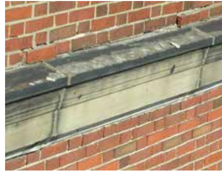
Loose brick due to poor conditions of mortar joints (moisture and movement in masonry system).
