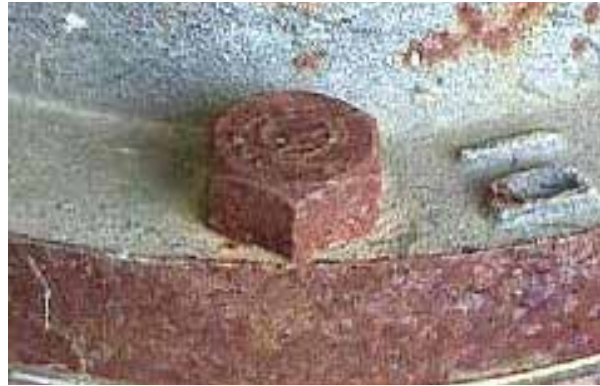
Galvanic corrosion resulting from a reaction between two dissimilar metals.
